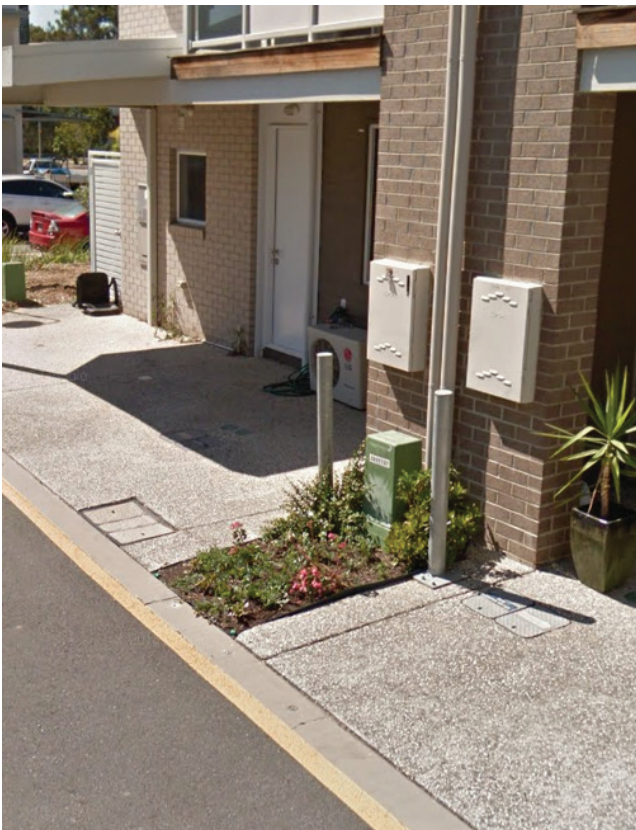
Figure 6.1.3 Laneway electrical service pillar with bollard protection
